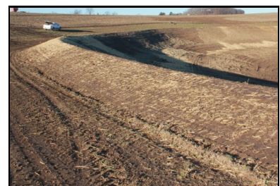
A water/sediment control structure traps sediment and reduces gully erosion. (Photo by Jacob Groth)
